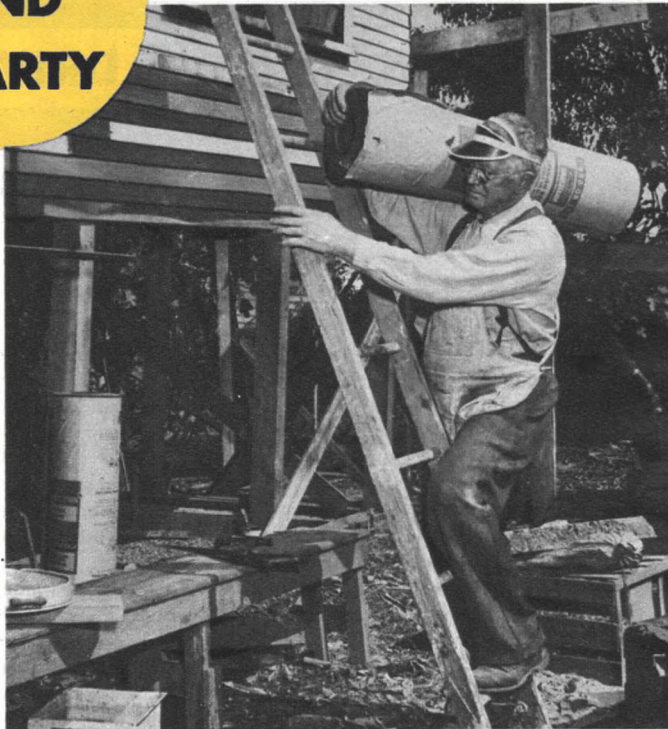
Jay W. (Daddy) Johnston, centenarian of Los Angeles, Calif., starts a roofing job as spryly as a youngster
